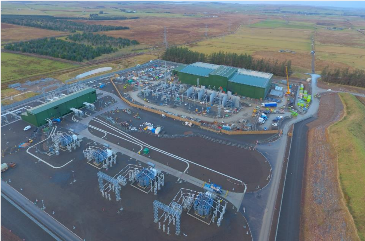
Spittal 800MW HVDC Converter Station
